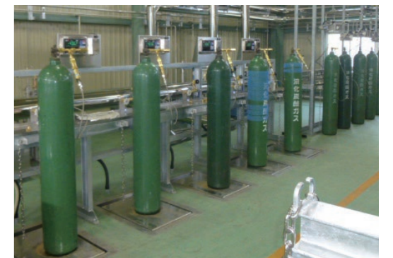
Gas reclamation and filling facilities
